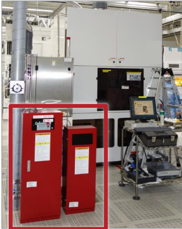
Automatic fire extinguishers
