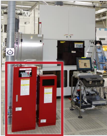
Automatic fire extinguishers
