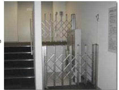
An elevator provides access to the roof at our Kitaitami Office
