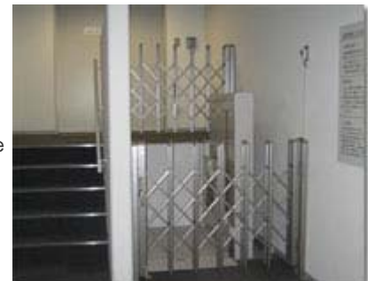
A platform lift provides access to the roof at our Kitaitami Site
