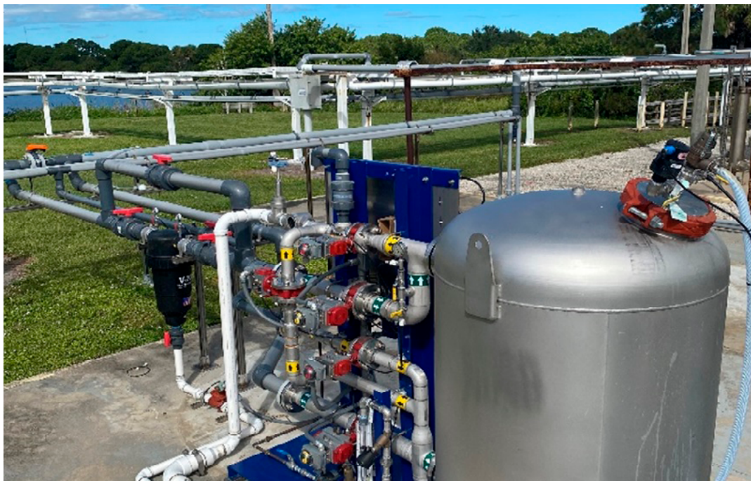
Reused water filtration equipment (Palm Bay Factory, U.S.)
