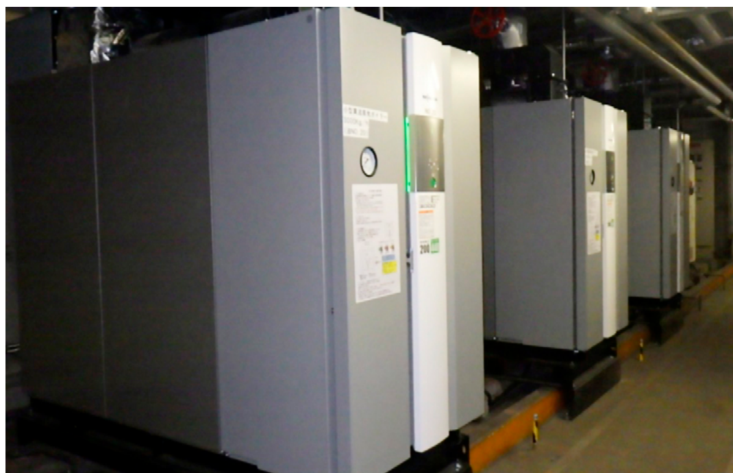
LNG-fueled boiler (Saijo Factory, Japan)
