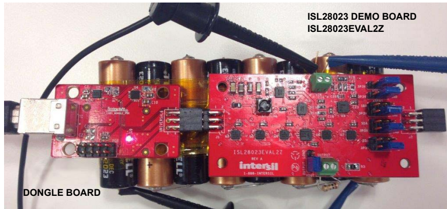
FIGURE 18. THE ISL28023 DEMO CONNECTED TO THE DONGLE BOARD AND A BATTERY PACK
