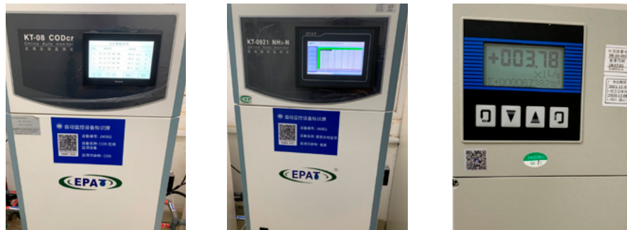
Online monitoring system of wastewater discharge
