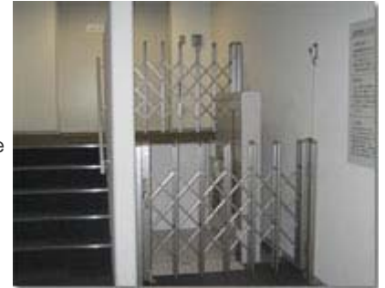
An elevator provides access to the roof at our Kitaitami Site
